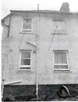
REAR OF PROPERTY Scaffolding required
